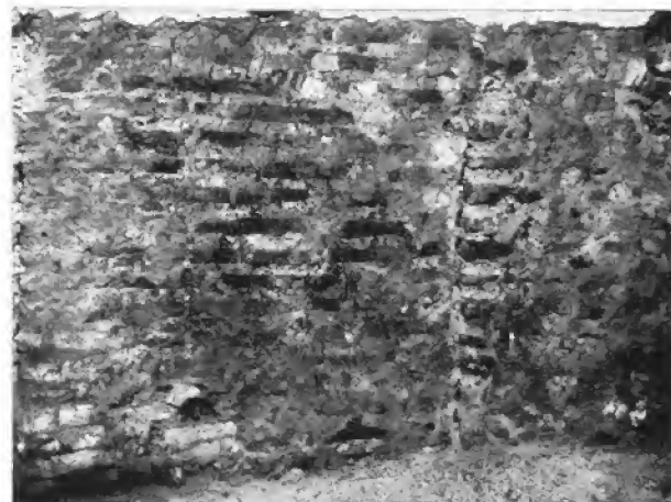
Fig. 149 — S. Lorenzo in Lucina. Right, core and internal brick face of original chancel wall. Left, secondary inner lining (Photo: Sansaini).
